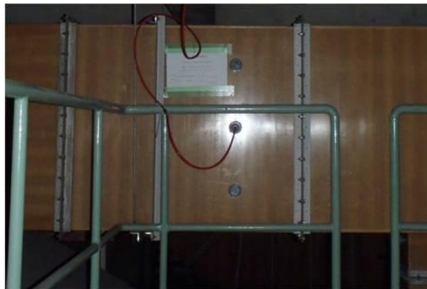
Exhaust Duct for Deodorization
